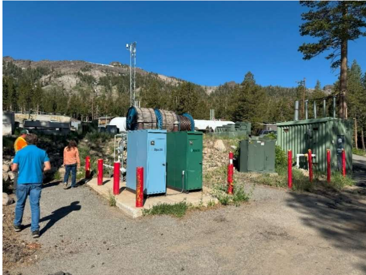
Figure 3.4: Existing Vaporizer (looking northwest)
