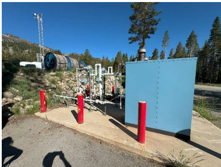
Figure 3.5: Existing Vaporizer (looking north)
